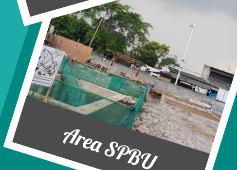
Under Ground Tank (UGT)
